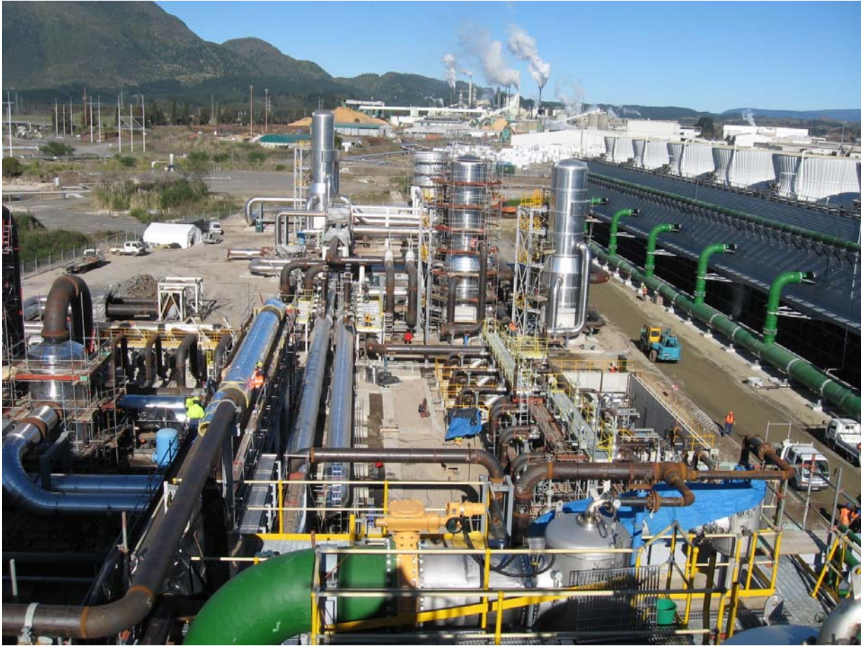
Mighty River Power's new 90MW geothermal power station at Kawerau nears completion (photo taken 9 June 2008)
